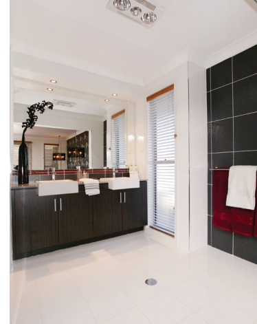
Figure 6.22 Heat lamps in a bathroom produce radiant heat, mainly through infrared waves.
